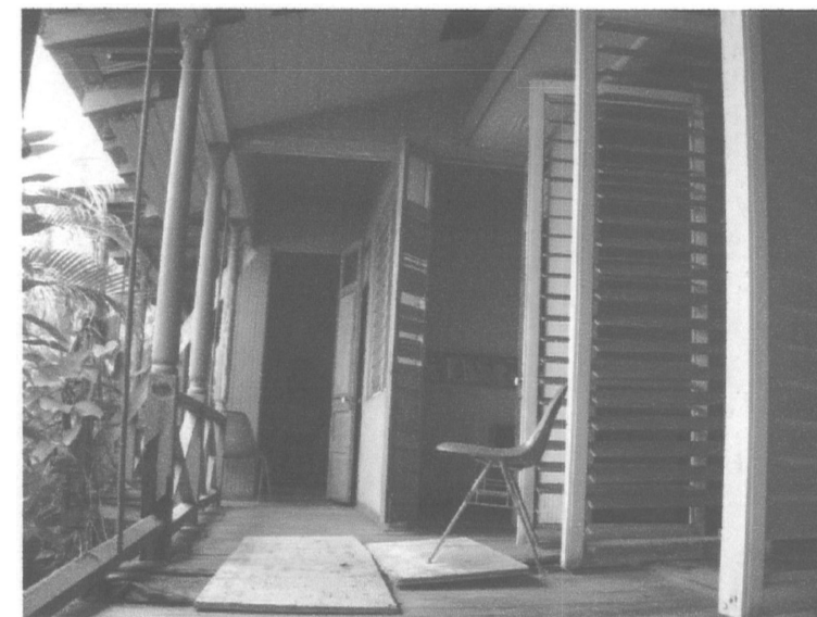
Figure 11: Casa Klumb / 2008 pivoting doors condition survey / AACUPR
